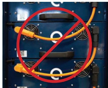
INCORRECT Cable is covering fan
